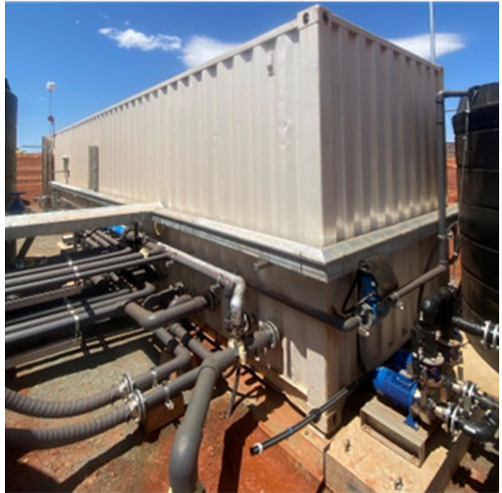
Dumbleyung Sewerage Treatment Plant
